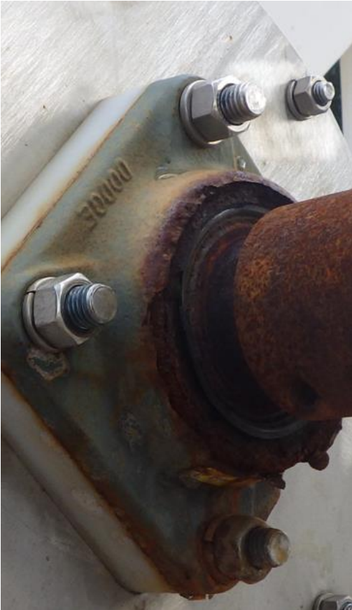
Clear evidence of failed bearing: outside corrosion, not lubricated
