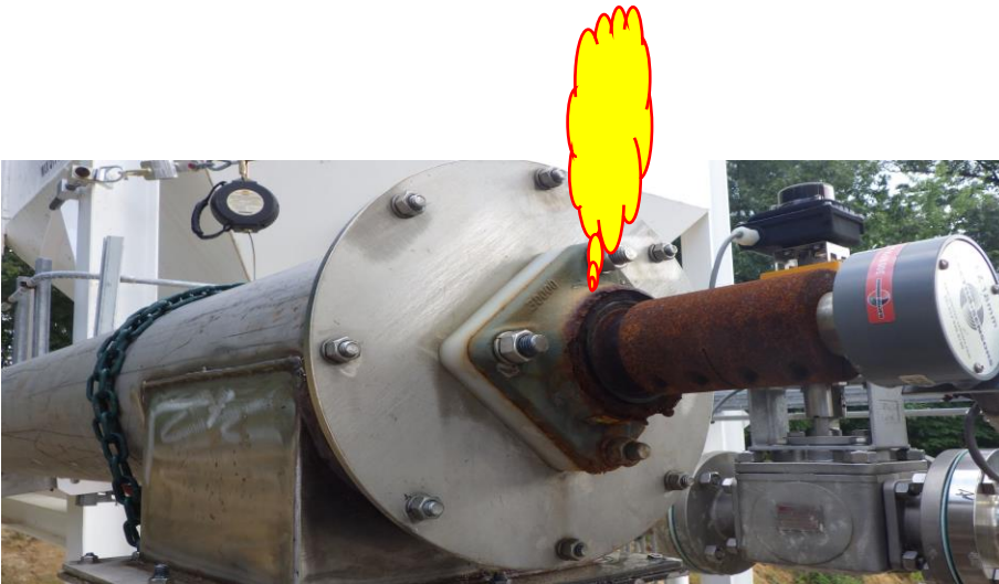
Place where smoke was detected
